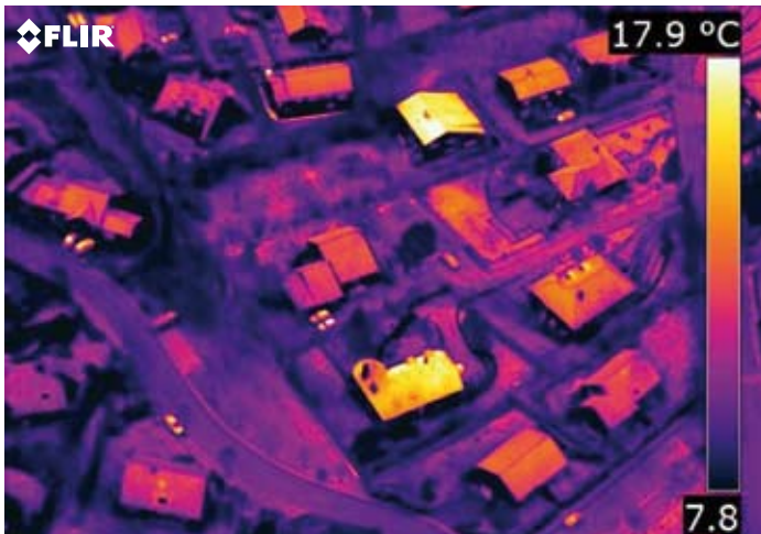
The buildings with yellow colored roofs show there is a moisture or insulation problem.
