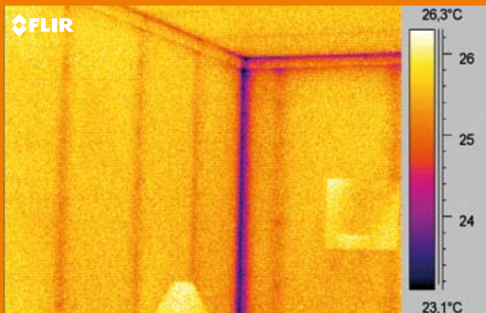
IR-image taken from the inside. The framework is visible, and so are the screws fitting the sheet covering to the framework. The corner is clearly colder, called a corner-effect, but there is nothing wrong here.
