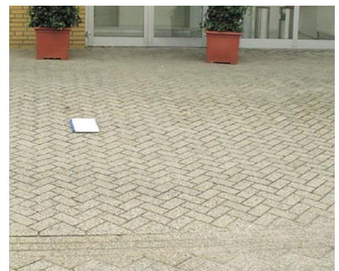
severe district heating pipe leak spotted by FLIR Systems S65
