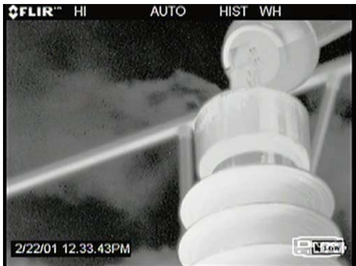
SF6 leak from a high voltage insulator
