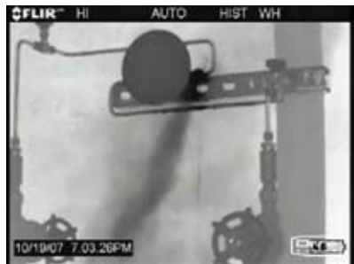
A leaking pressure gauge
