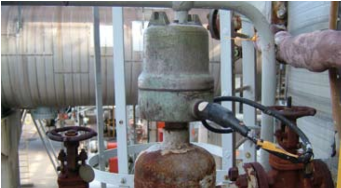
Level float switch
