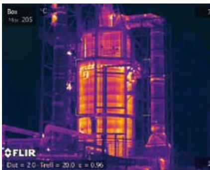
Infrared image of a process furnace
